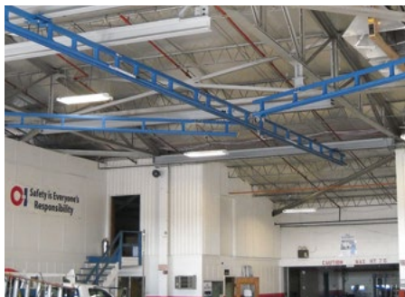
CEILING MOUNTED MONORAIL
